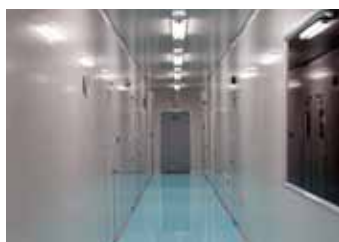
API Finishing Area
