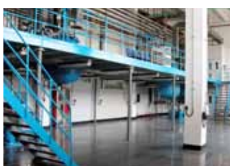
Pilot Plant Area II
